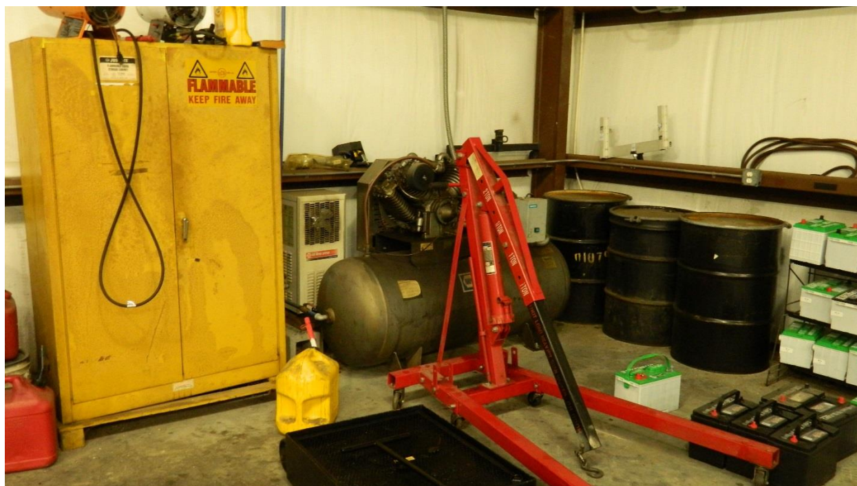
Air Compressor – Tract A
