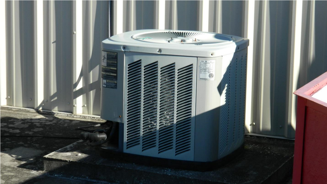
Heat Pump that Cools/Heats Office – Tract A
