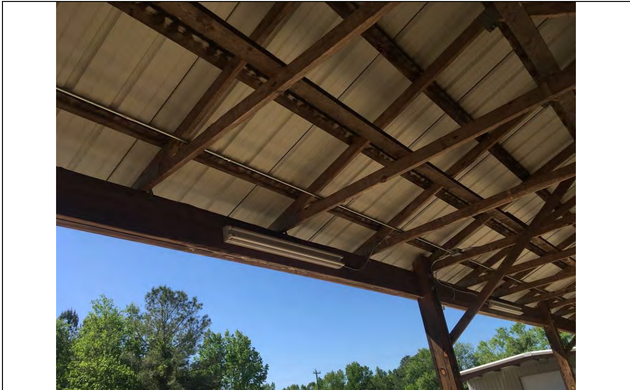
Photo 7: Water staining on underside of roof supports indicates some existing leaking of roof
