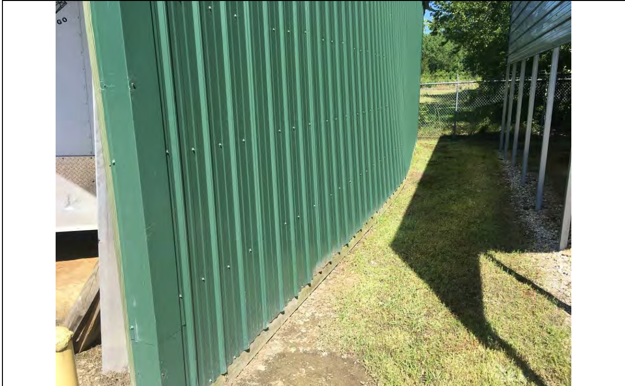
Photo 6: Most severe damage along north side resulting in distortion of north wall
