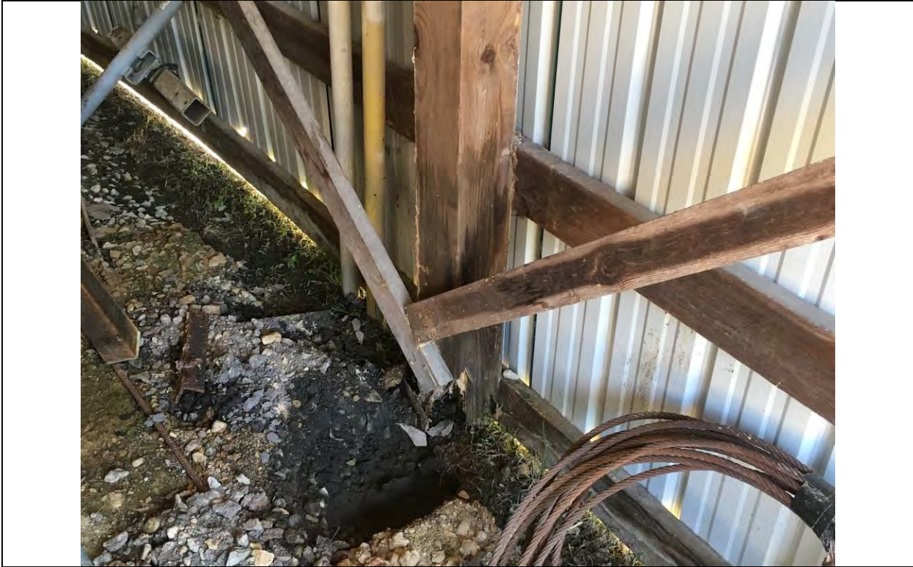
Photo 4: Timber support at north wall completely detached due to termite damage
