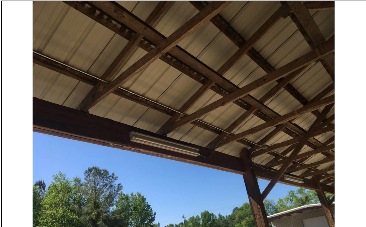
Photo 7: Water staining on underside of roof supports indicates some existing leaking of roof
