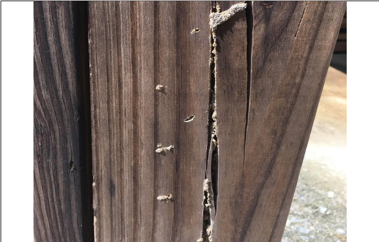
Photo 3: Evidence of termite presence inside timber support post
