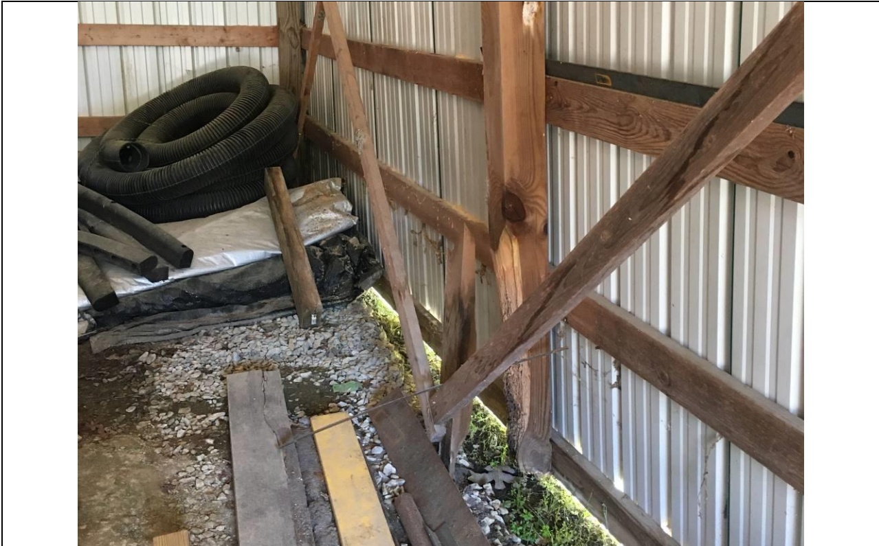
Photo 5: Timber support at north wall completely detached due to termite damage
