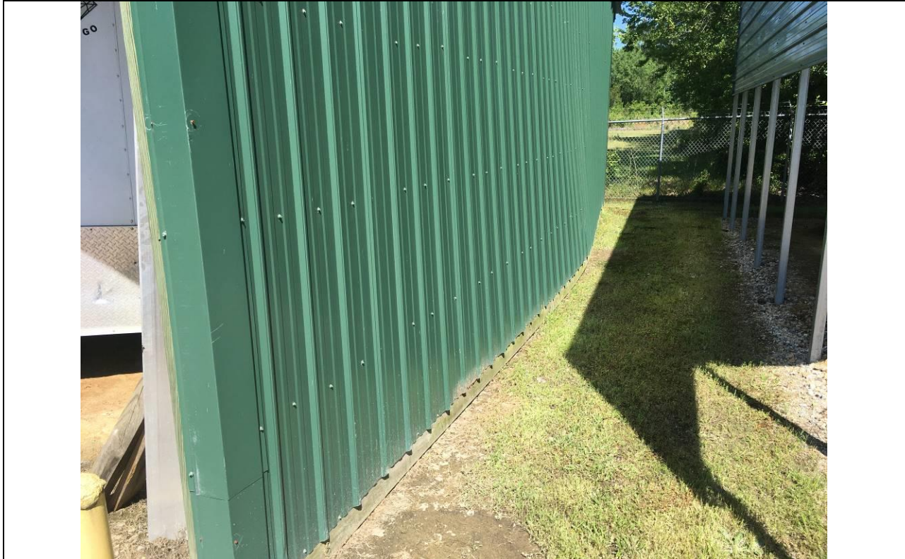
Photo 6: Most severe damage along north side resulting in distortion of north wall
