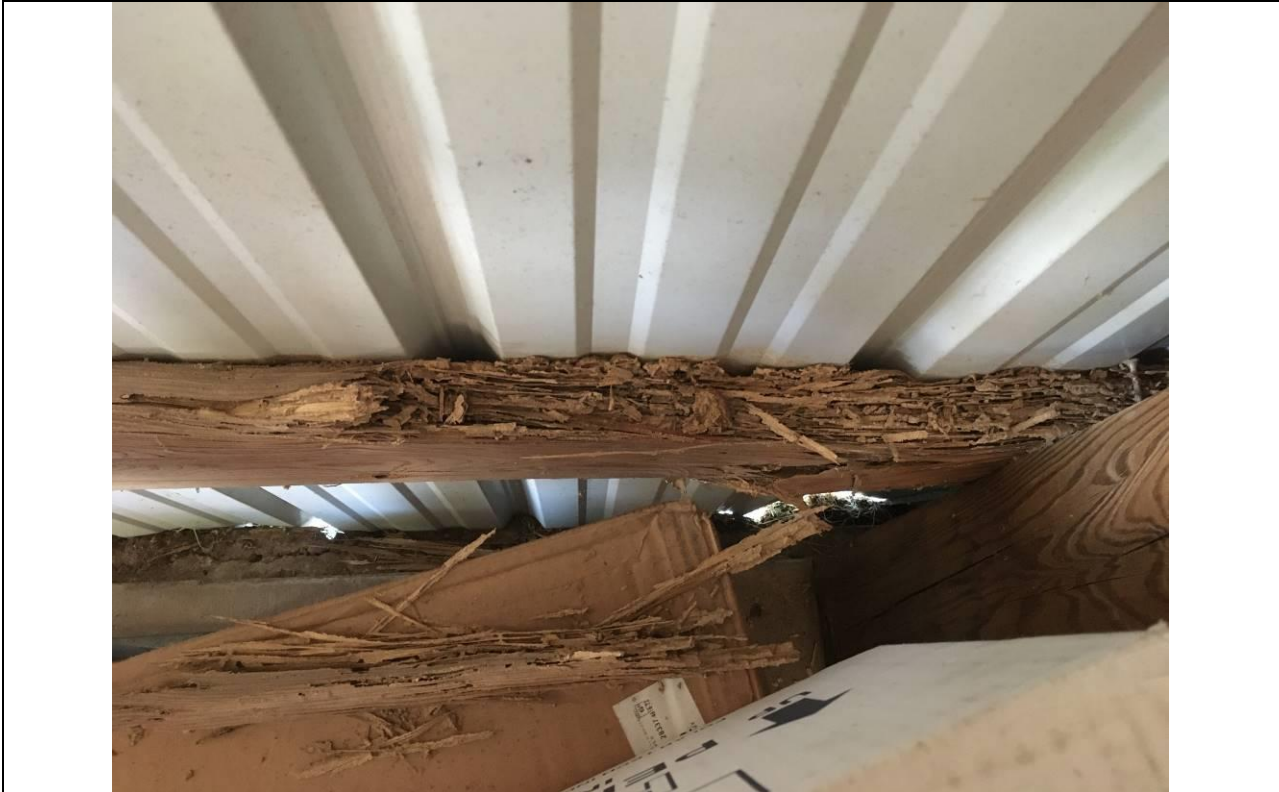
Photo 2: Severe termite damage of timber girt that provides bracing and attachment point for siding
