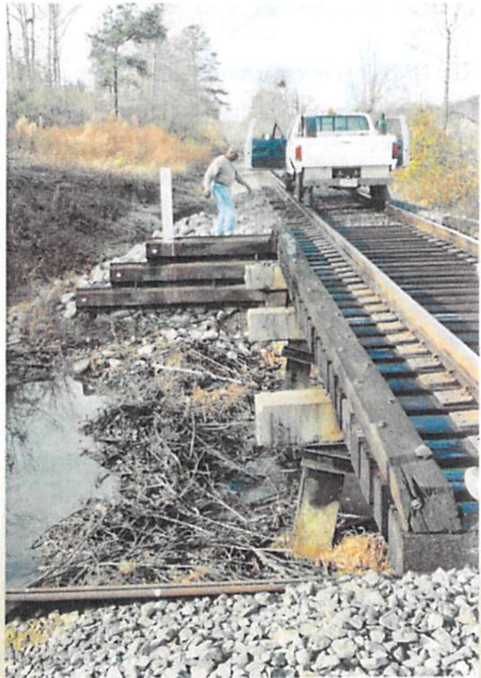
Beaver dam blocking a CSX railroad trestle in Wake County. In February 2000, 39 cars of a CSX train carrying hazardous chemicals derailed due to a collapsed trestle in Pitt County. Backed up water from a beaver dam eroded the railroad bed and was blamed for the wreck.
