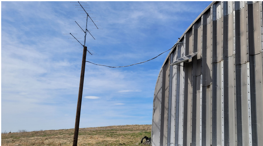
Antennas are mounted on the wood pole and the receiver station is housed inside the hangar, safe from the elements. (Chris Kelly)
