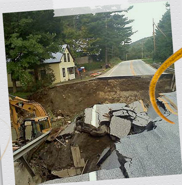
Damage from undersized culvert failure
